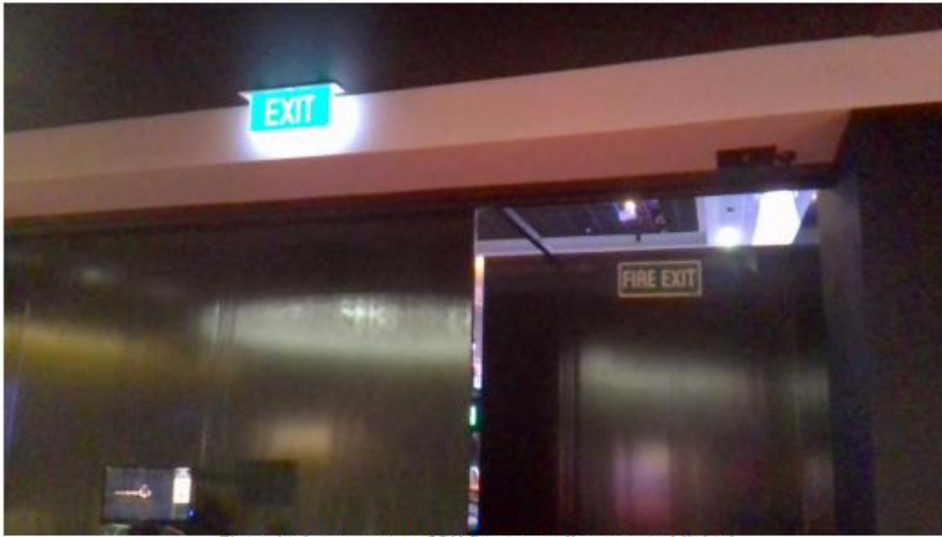
Fire exit signage as per CPU fire report diagram established Taken at 11:14 AM on Tuesday 15/04/2025
